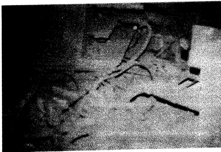
No. 9 Damaged power center 6 Right North
